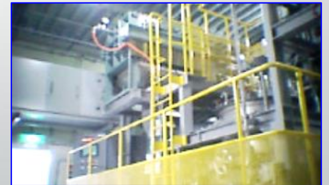
Miscellaneous solids reduction mortar solidification device
